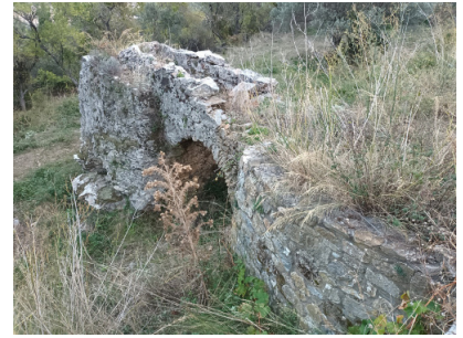
Fig. 4. The drop tower (funnel-shaped cistern) and part of the mill race, which is supported by an arch (photo by I. Papaeftychiou).
