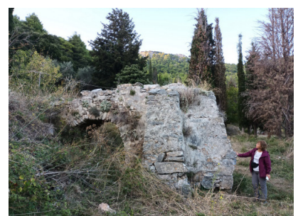
Fig. 8. The large buttress supporting the drop tower of the watermill, on its south side (photo by I. Papaeftychiou).
