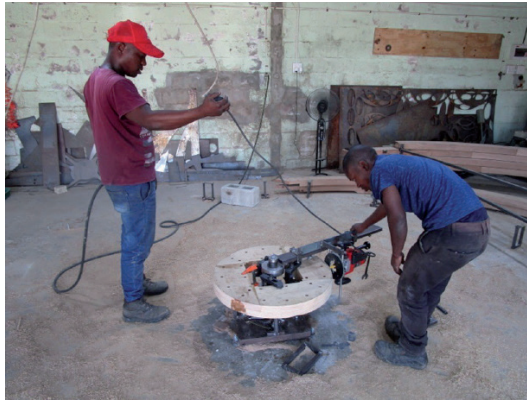
Pinion disc being machined on the same radius jig that the curb, cap ring and brake wheel were made on.
