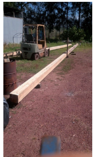
Two 8m beams laid end to end. Now they must be joined!
