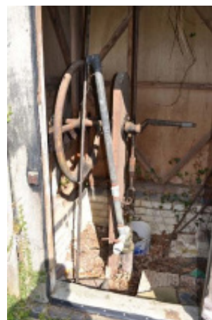
The borehole pump, which can be driven by wind or by hand (both photos May 2016).
