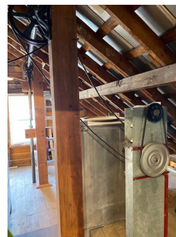
Another view of elevators, bin and drive.
