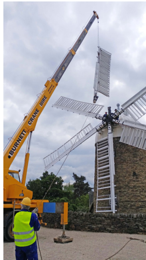
The last of the sails is lowered into place by the mobile crane.
