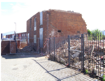
Photograph 11 taken 5th August 2017: Work moved only slowly down to the ground floor.
