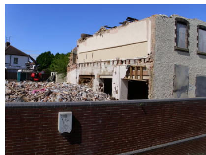
Photograph 12 taken 5th August 2017: And the same at the rear.
