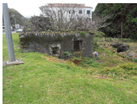
Fig. 1. Watermill near Sao Vincente, on the north coast. It is ruinous and uncared for and at the edge of a modern traffic roundabout. Still with a very good pair of millstones inside, fighting for space with a big fig tree.
