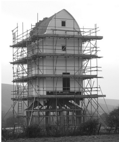
Ashcombe Mill during its re-construction. The steel framework can be seen in the mill's round-house.
