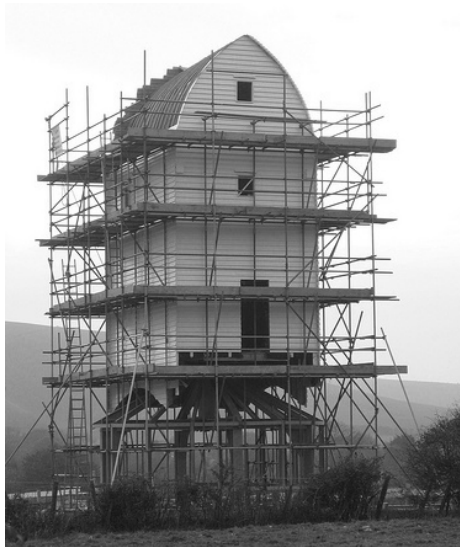
Ashcombe Mill during its re-construction. The steel framework can be seen in the mill's round-house.
