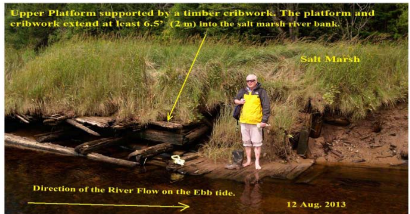
Two platforms at the Apple River watermill site. The upper platform is 2' (0.61m) above the lower platform. The man in the photograph is Professor David Patriquin, retired from Dalhousie University, Halifax, Nova Scotia
