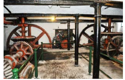
The main drive shafts and gearing
