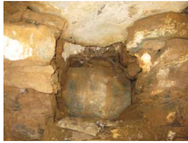
The blocked hole inside the kitchen for the chicken to be able to come and go
