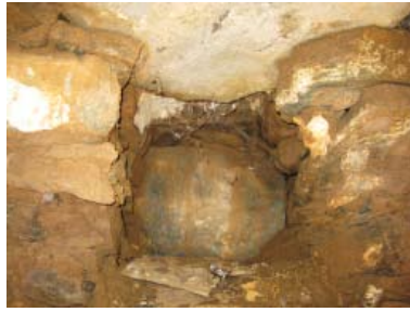
The blocked hole inside the kitchen for the chicken to be able to come and go
