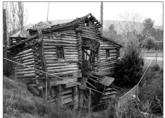
Fig. 2. Hart Park waterwheel today, partly collapsed and surrounded by a safety fence.
